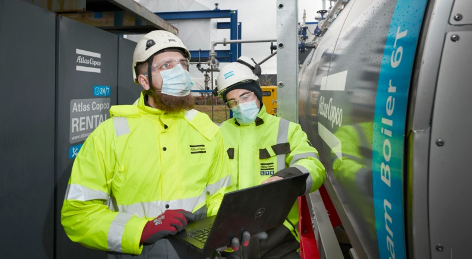
24t/h superheated steam solution including boilers, feedwater tank, steam manifold, steam silencer and lines in a chemical plant.
